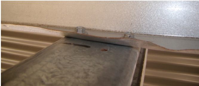
Poor support conditions (flange not sitting flat).
