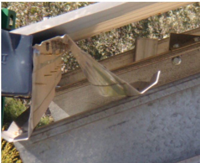
Spread of TOPSPAN® During Incorrect Installation.
