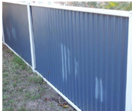
Figure 2. Irregular faded appearance of touch-up paint on fencing panels
