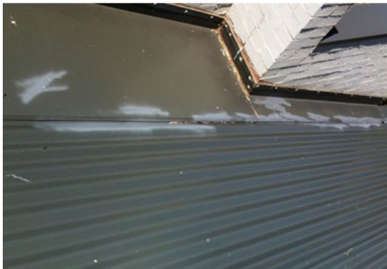
Figure 1. Irregular faded appearance of touch-up paint on roof flashing and roofing broad sheet
