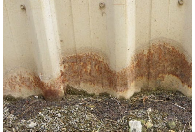
Figure 3. Corrosion due to immersion in soil
