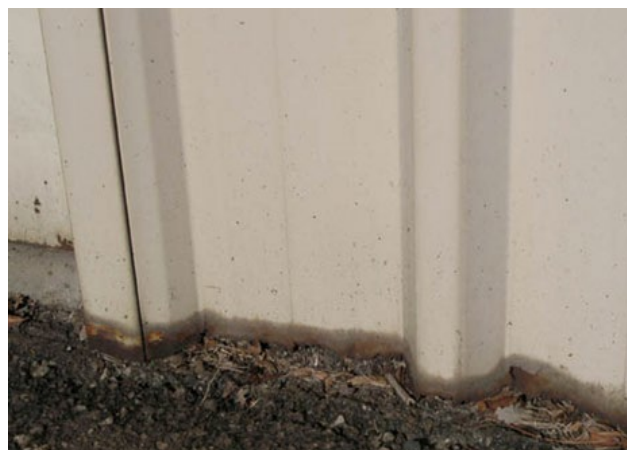
Figure 2. Corrosion due to inappropriate wall design
