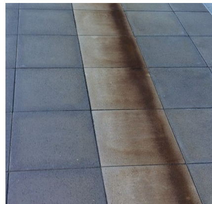
Figure 2. Concrete staining due to incorrect management of runoff from weathering steel wall directly above
