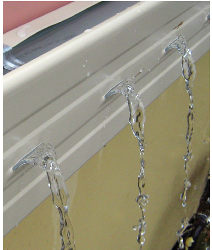
Typical overflow from slotted gutter.
