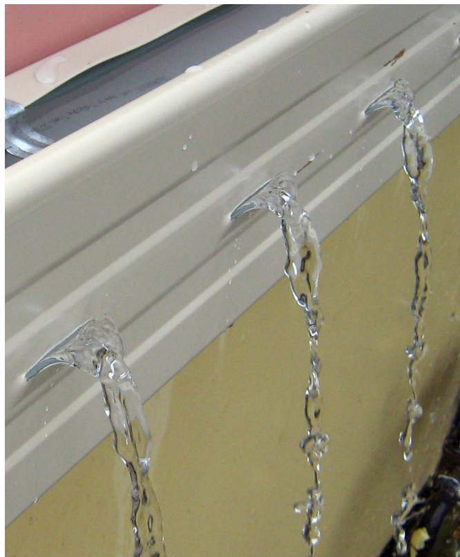
Typical overflow from slotted gutter.
