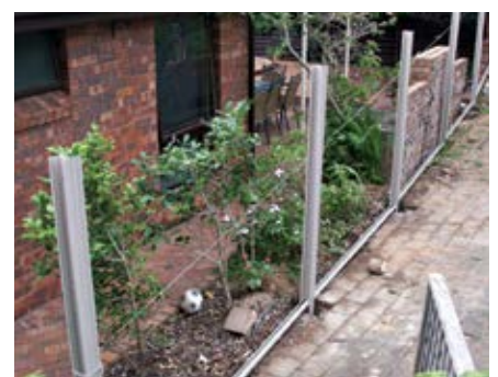
Set all the bottom rails into position ensuring a 50mm ground clearance.
