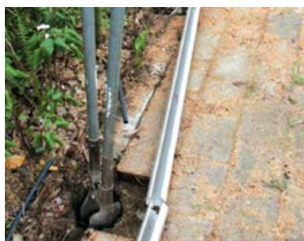
Lay the rails along the string line to determine positions of posts.
