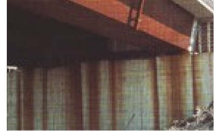
Figure 3.12b Bad detailing (severe staining) [Image courtesy of TxDOT]
