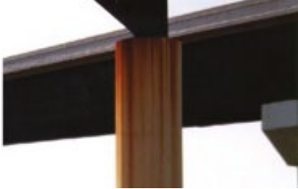
(a) Concrete column without protection of drip pan
