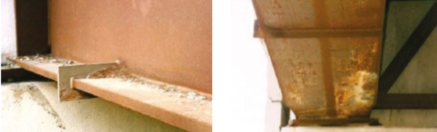
Figure 3.13 Bad detailing of drip plate. Drip plate improperly set at 90°, creating corner for debris accumulation (left); and Drip plate not set at proper angle (right). [Images courtesy of TxDOT]
