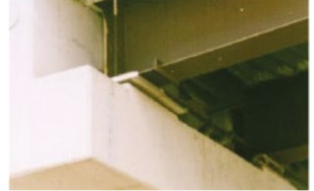
(c) Stain-free concrete due to installation of drip plate
