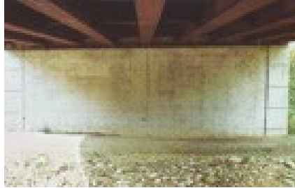
Figure 3.12a Good detailing producing an abutment free of staining [Image courtesy of www.steelconstruction.info]
