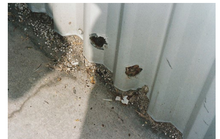
Figure 1: Corrosion due to fertiliser contact
