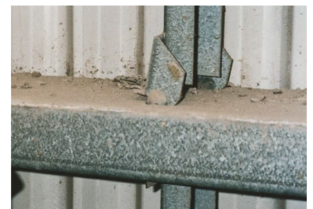
Figure 2: Build-up on purlin
