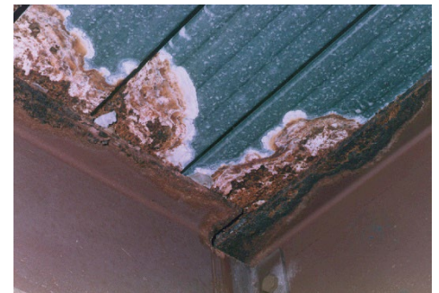
Figure 1: Corroded concrete decking showing the result of sub-standard expansion joint and finish detail
