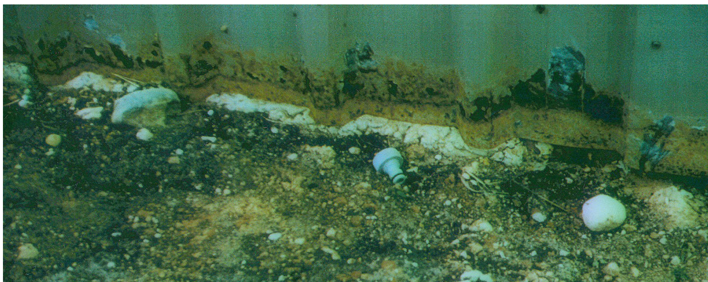
Figure 1: Immersed Shed Wall
