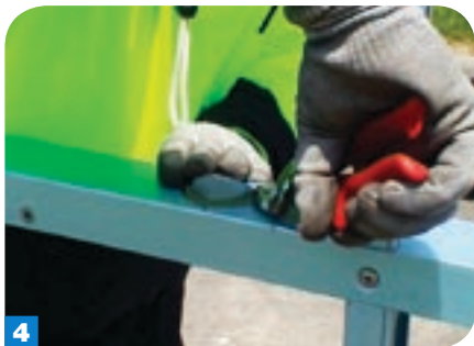
4 If the hole is too close to a stud, you'll need to change to the other snip to finish the cut from the other direction to avoid the stud interfering with the progress of the snips.
