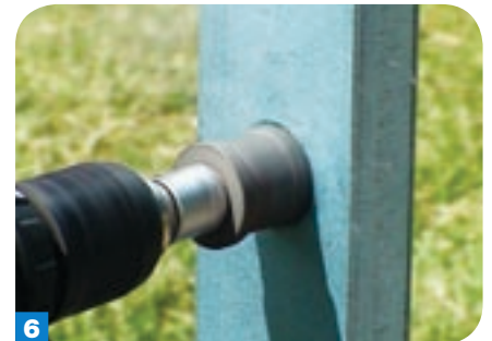
6 A larger pilot hole is required for the bigger mandle. In this case, use a water pipe-size punch or cutter.
