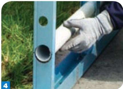
4 The same hydraulic tool is used to make smaller holes for water pipe and electrical cable.
