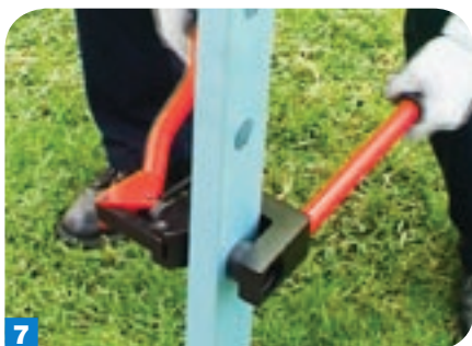
7 A hand punch for light gauge steel is used to create the pilot hole.
